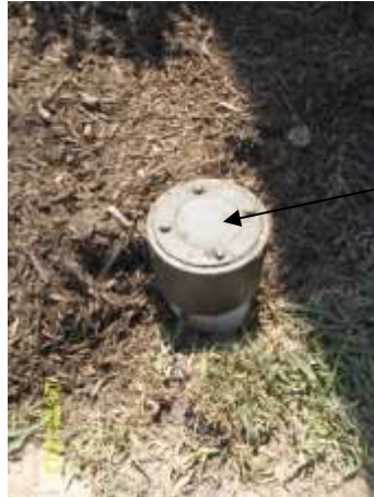
Pop up cover keeps the sewer from backing up into the home in this example photo
